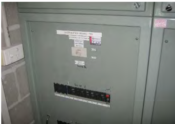
Photograph 17. Loading Dock level S: Main Switch Room No.1 - Electrical Sub-cabinets, Main Isolator and D.B services - Non-asbestos E.M.B's
